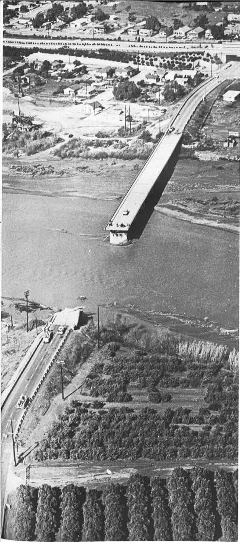
The Willard Bridge over the Santa Clara River in Santa Paula was left in ruins by January's storm. When the bridge went out on Jan. 25, it helped to isolate the city of Santa Paula. Residents were marooned for about five hours.
