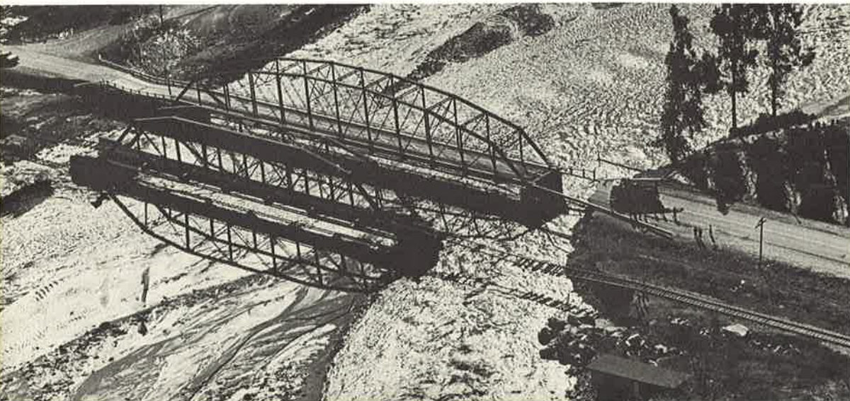
Bridge at junction of Old Telegraph Road and Grand Avenue in Fillmore, left, was washed out during January storm, cutting off the bridge approaches and Southern Pacific Railroad route to Newhall. Below, flood waters cut a wide swath through a county citrus grove. Crop damage from floods ran into millions of dollars.
