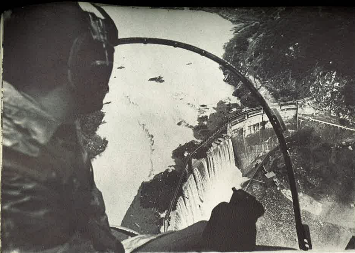
Helicopter pilot, Grady Ragsdale, Jr., watches torrents of water flow through the notch cut in the top of Matilija Dam.
