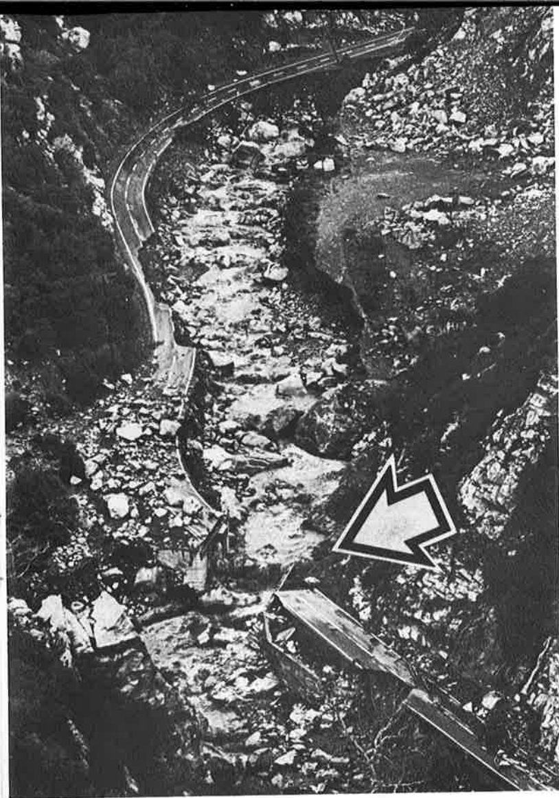
Portions of Highway 33, at left, were all but obliterated by January's storm. Parts of the highway which escaped raging river waters were severely damaged by rock slides.
