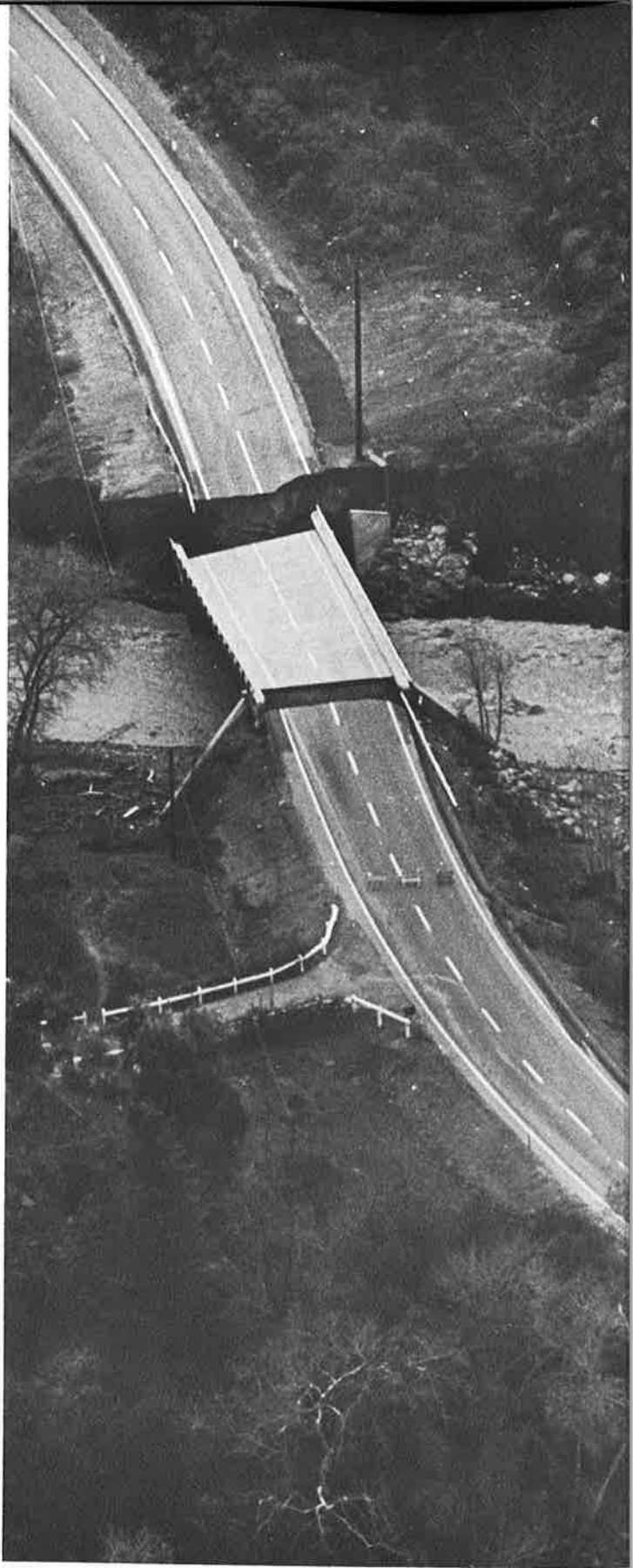
The Highway 150 bridge that spanned Santa Paula Creek near the entry to the Ferndale Ranch at Sulphur Mountain Springs did not quite make connections after January's raging storm. It will take months to repair damaged roads.
